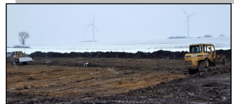
Crews install two water-and-sediment control basins in December at a Clayton Township farm in Mower County for the Root River Field to Stream Partnership.
